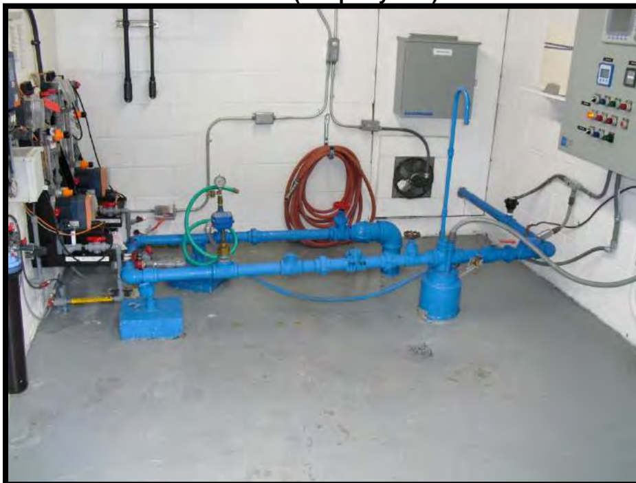
Well S24 (Nisqually 19A)
