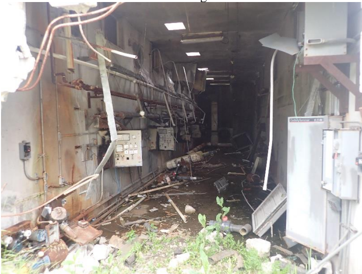
Photo 17. Mushroom farm mechanical building
