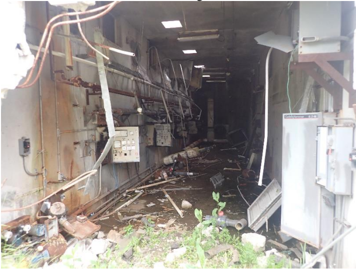
Photo 17. Old mushroom farm mechanical building stripped
