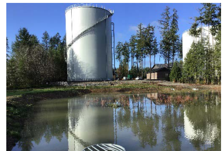
Second reservoir added to support maintenance and redundancy, existing detention storm pond modified to handle additional impervious surface at Hawks Prairie Reservoir
