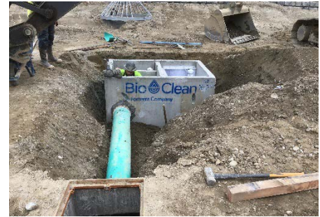
New stormwater system tying into a new filter vault to treat the added impervious surface associated with the Hawks Prairie Reservoir "Sister Standpipe" project
