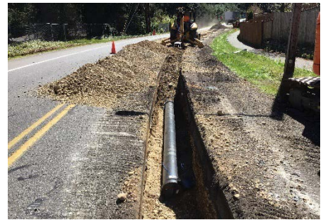
Installing a new water main and valves/appurtenances as part of the water replacement utility improvements at Carpenter Rd
