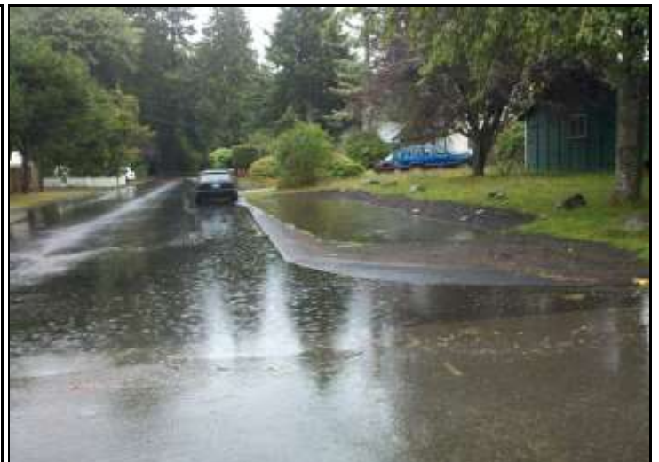
Road without drainage system
