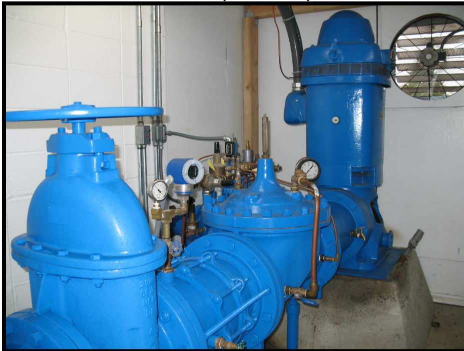
Well S07 (Fire Station)
