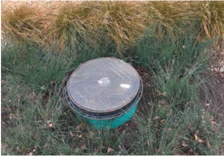
Underground Injection Control (UIC) Well
